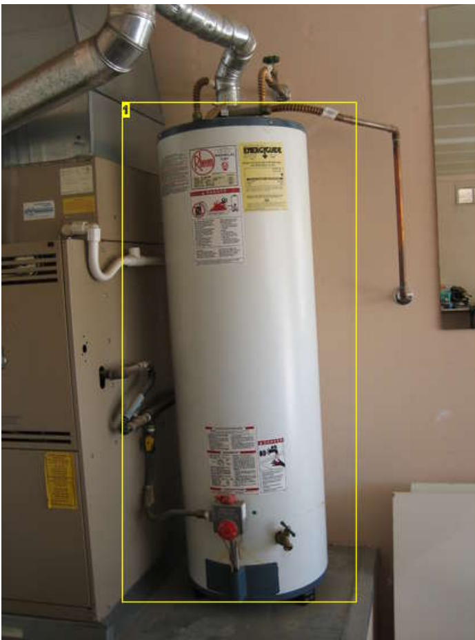
Image Notes 1. Water Heater
