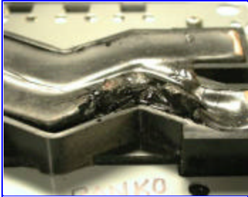
FIGURE 3 - OVERHEATING AT THE CONTACT BETWEEN THE BUSSBAR AND THE STAB SOCKET ASSEMBLY CAUSED THIS DAMAGE TO THE INSULATION. [Click for larger picture]
