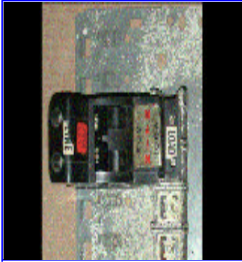
FIGURE 6 - FPE 100-AMP MAIN BREAKER CONNECTS TO THE BUSSBARS THROUGH THE PLATE & POST CONFIGURATION, USING ONE 8-32 SCREW AT EACH TERMINAL.
